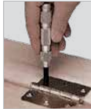
Punch being used to mark screw starting centres on a door frame
